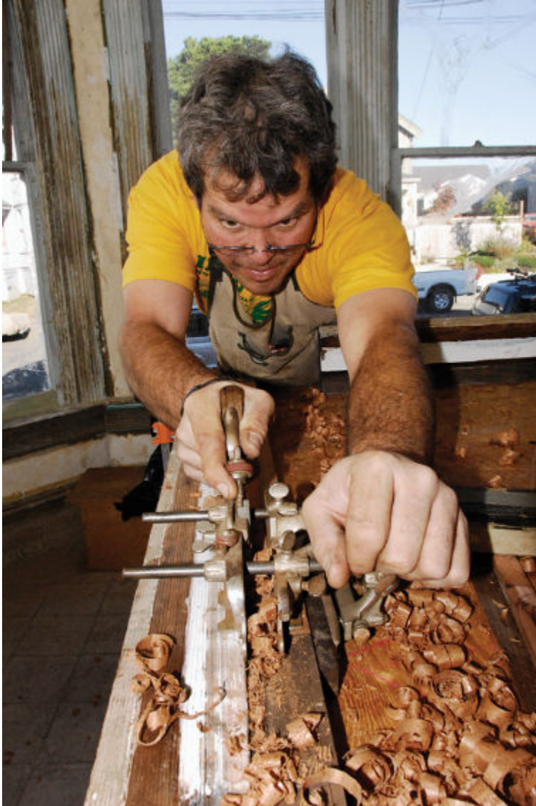
Bill Hole, CR professor of construction and historic preservation technology, repairs on an old window frame at the Annie B. Ryan House. Hole's Field Technologies class works on the house each Saturday. Joni Schrantz/The Eureka Reporter
